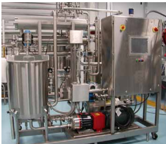
The pilot skid system installed at the Ecolab R&D Center allows for 24/7 testing and troubleshooting of all standard spiral membrane sizes, at all relevant pressures and all pore sizes from MF to RO.
