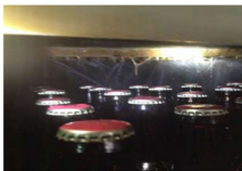
Mesh is blocked by microbial slime, and nozzle is partially blocked, Uneven water flow due to blockage of the nozzle part
