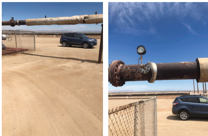
Picture 1&2: Target area to setup the containment basin, totes, pump, and tubing (left). Target area to inject the quill for the chemical application point (right).
