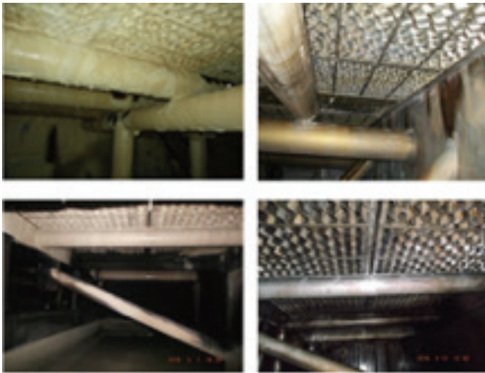
Image 1 - Barometric condenser fill, before and after chemical cleaning
