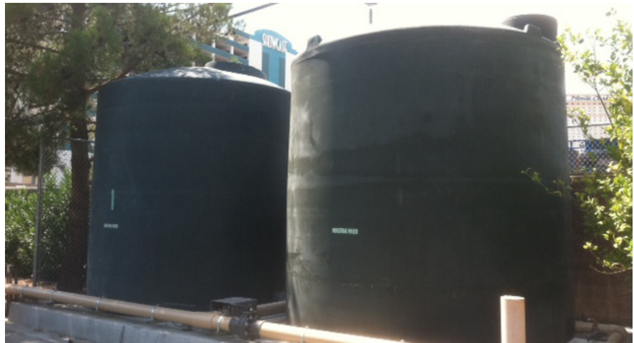
Well Tanks Close Up
